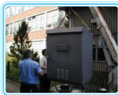
NEMA Control Cabinet
